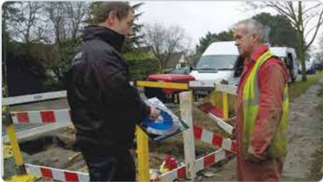
Service & support on site
